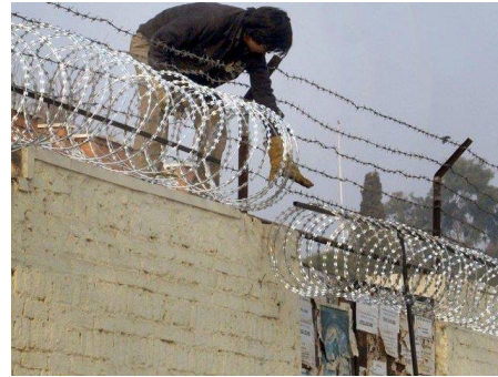
The erection of concrete walls and barb wires seen throughout the city especially in front of schools, college and institutions. Source: The Express Tribune
