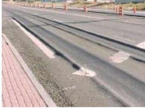
Figure 2.13: Severely rutted road (Dynamic Shear Rheometer, n.d.)
