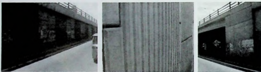
Fig. Concrete on the ramp wall; the vertical pattern of the concrete panels, The texture of a single concrete panel, Breaking of the pattern with a exposed concrete panel, the illustration of the visual properties of the panel.
