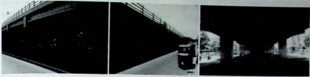
The structure of the flyover; the space created with column structure, The solid ramping unit, the space under the flyover.
