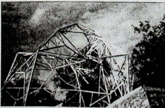
Fig 1 Beliaththa 70m antenna tower collapse
