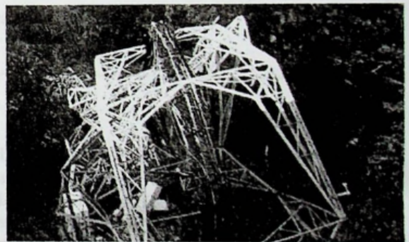
Fig 4 Horowpathana 70m antenna tower collapse
