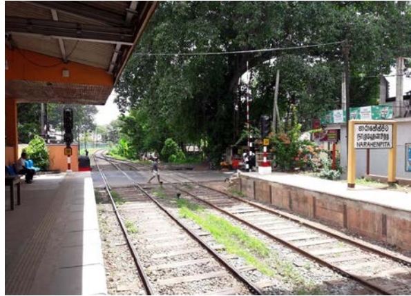
Figure 4: New Signalling system at Narahenpita
