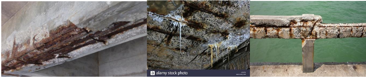
Figure 8: Reinforcement steel bar corrosion because of the high permeability of concrete
