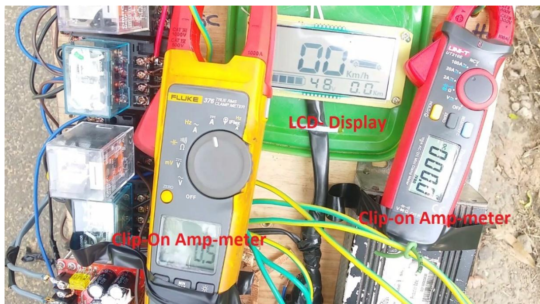
Figure 5.2.1 On-load test arrangement
