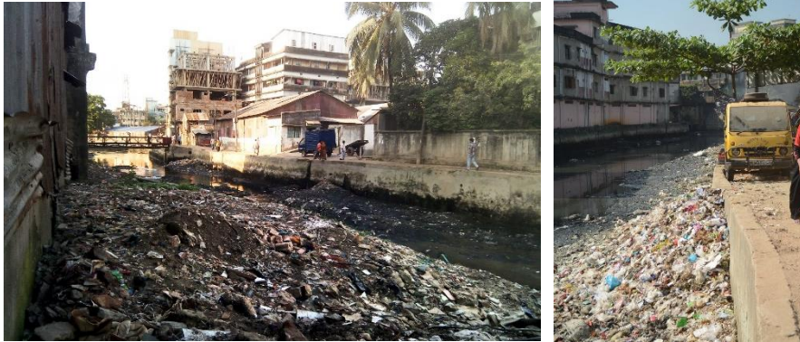
Figure 3, Garbage Disposal along canal front blocks canal (Source: Author)
