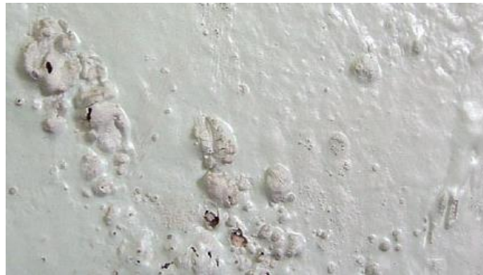
Figure 1.2: Damage surface due to Efflorescence
