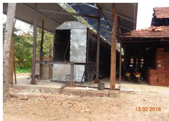
Figure 7 : Trolley and heat pipe arrangement in the dryer
