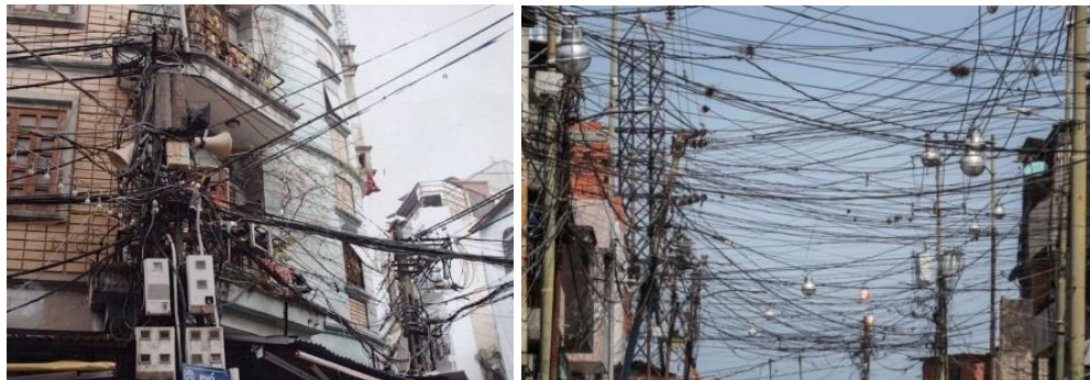
Figure 13: Hanging wires Source: https://www.google.com
