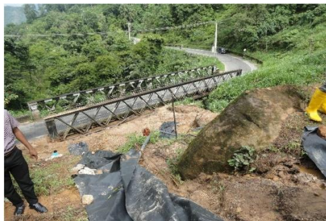
(e) Unstable boulders
