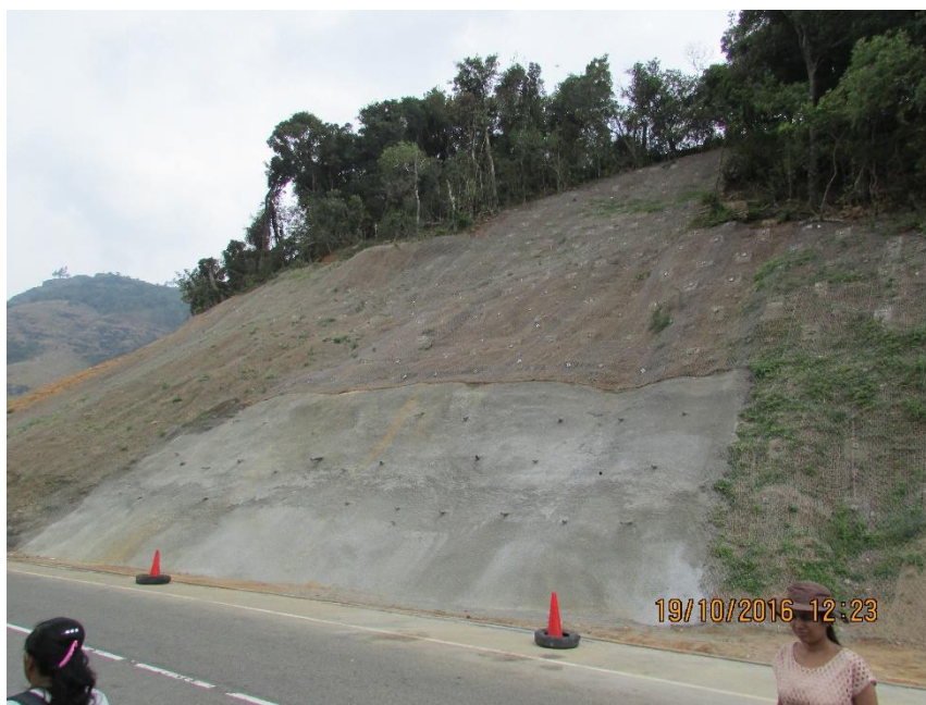
Figure 2.34 : Mitigation Measures with Soil Nailing and Facing with Individual Pillows Connected by High Tensile Wire Mesh, and Vegetation
