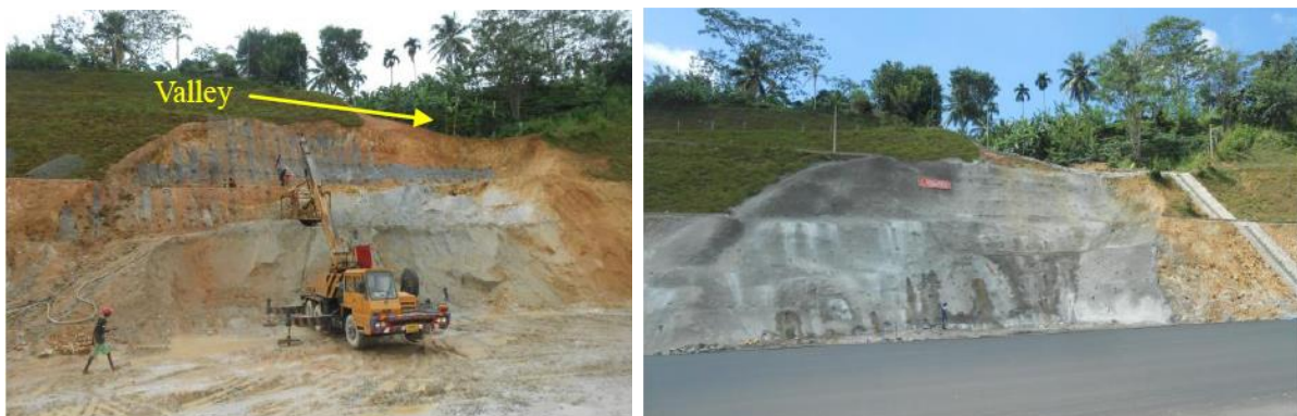
(a) After Failure (b) After Rectification Figure 2.35 : Failure at 41 km on Southern Expressway Extension
