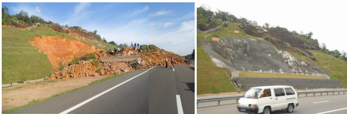
(a) After Failure
