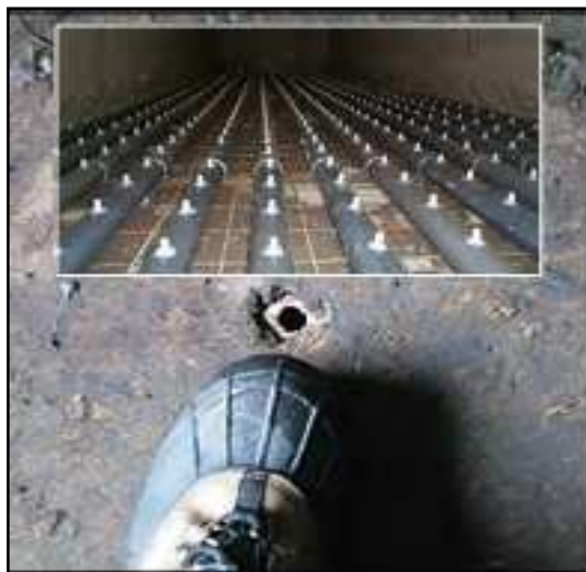
Figure.2.47: In-floor aeration with pipe and spigot system; inset photo shows system prior to concrete floor being poured[17]
