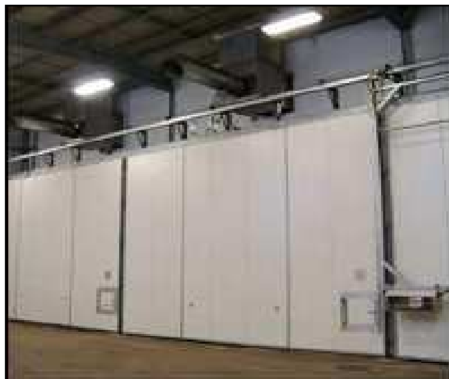
Figure.2.53: Close up of tunnel door system [17]
