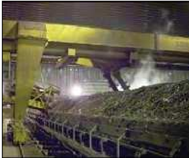
Figure.2.62: Bridge crane and suspended auger turning mechanism viewed from discharge side of Bay[17]
