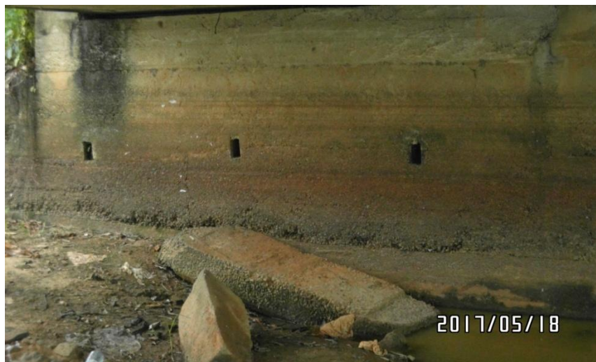
Figure 3-23: Weathering of cover concrete in an abutment wall
