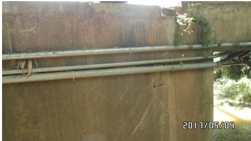
Figure 3-20: Cracking at wingwall due to lateral earth pressure
