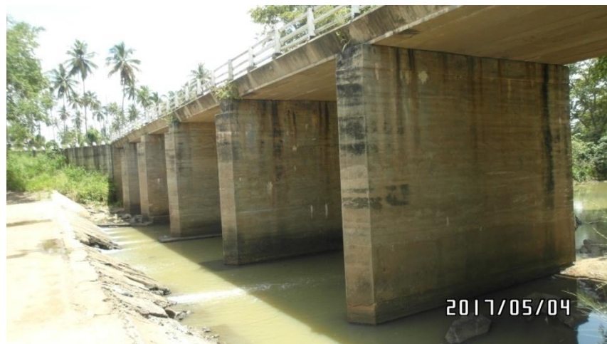
Figure 3-16: Leaking through expansion joints
