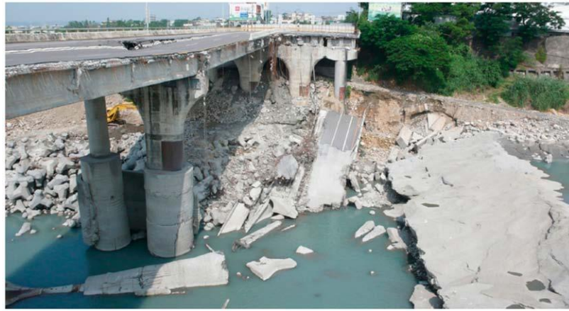
Figure 2-2: Collapse of Hou-Fong Bridge, Taiwan in year 2008 [5]
