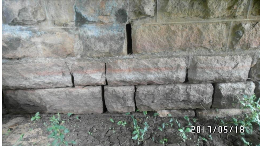
Figure 3-18: Dislocation of mortar at an abutment wall
