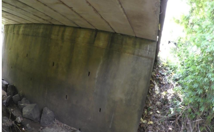
Figure 3-21: Vertical crack at a RRM abutment wall due to settlement
