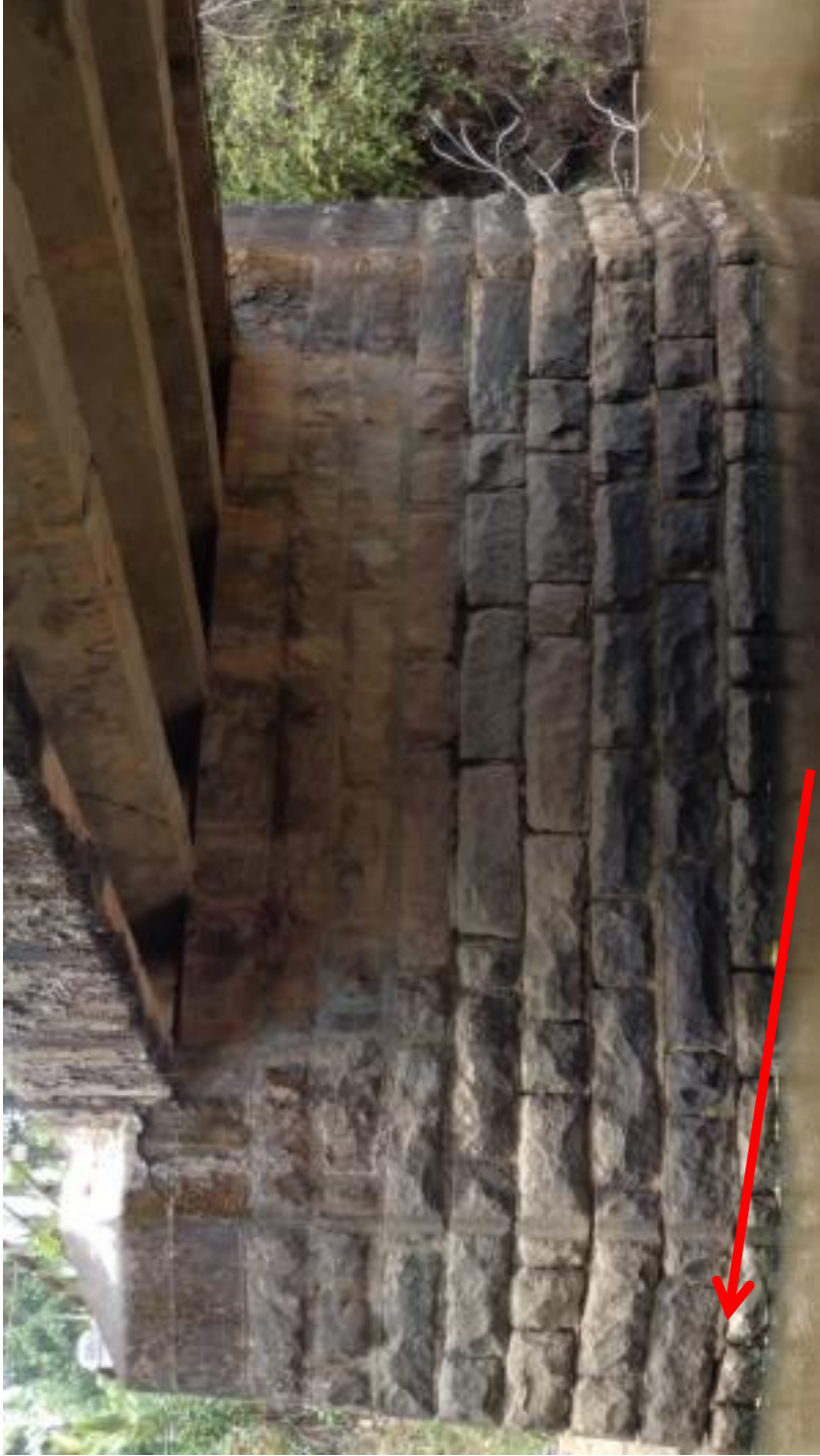
Mortar dislocation due to water pressure at upstream
