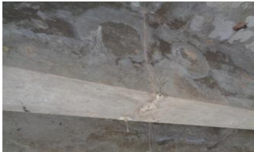
Figure 3-9: A flexural crack on a bridge beam
