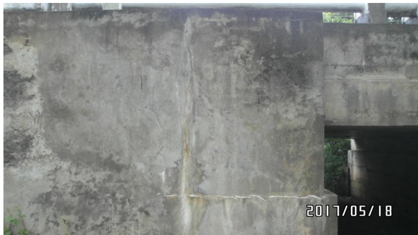
Figure 3-11 : Map cracking due to moisture movement
