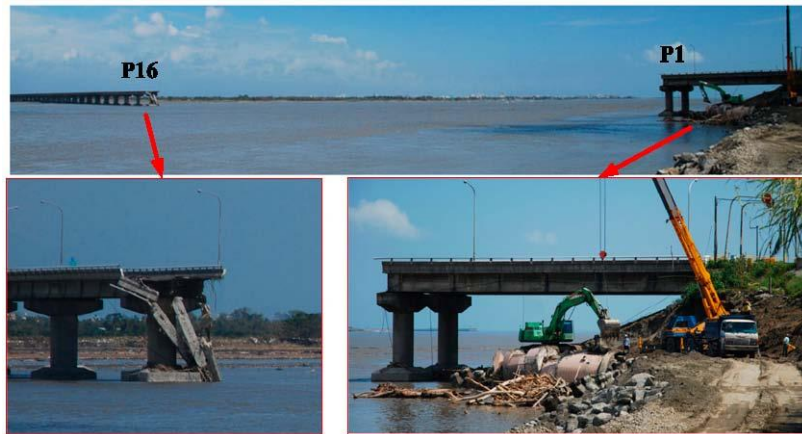
Figure 2-3: Collapse of Shuang-Yuan Bridge, Taiwan in year 2008 [5]
