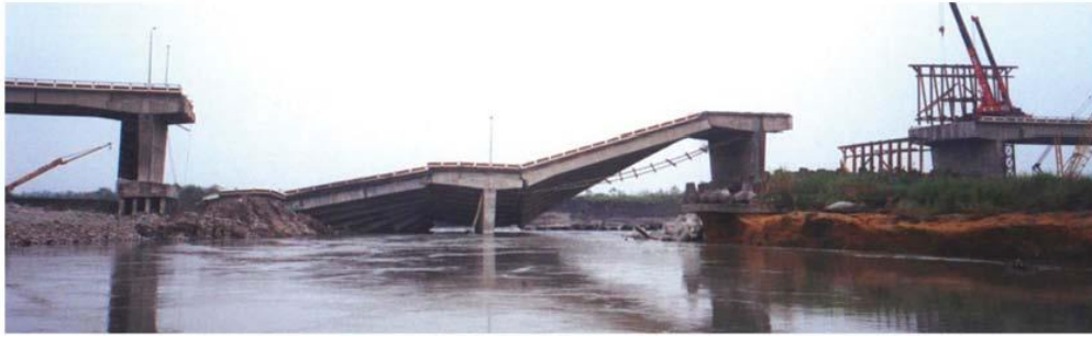
Figure 2-1: Collapse of Kao-Ping Bridge, Taiwan in year 2000 [5]
