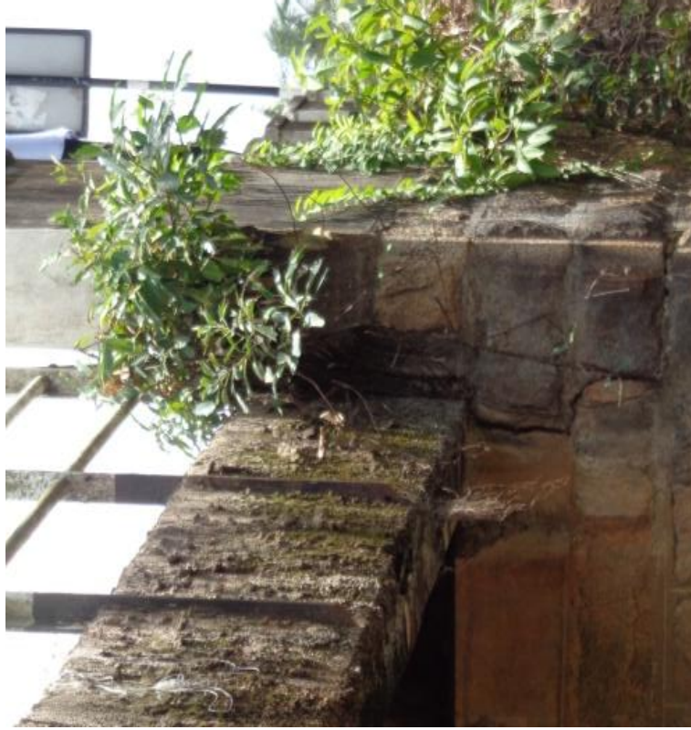
1 - Crack due to lateral earth pressure
