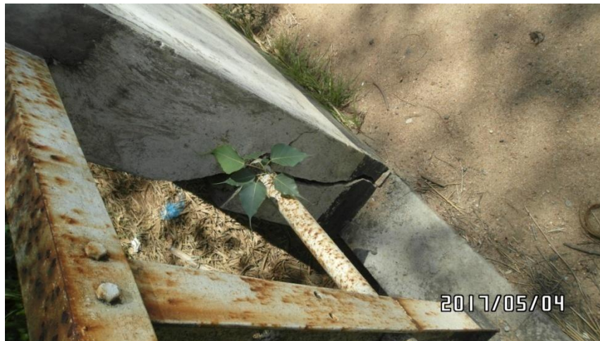
Figure 3-14: Effect of vegetation at an old handrail
