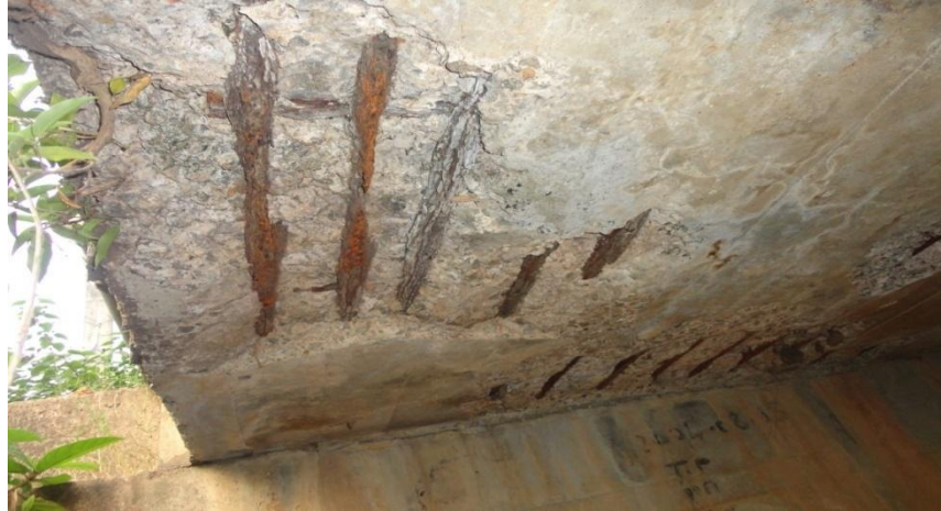
Figure 3-6: Corrosion of reinforcement underneath a slab bridge
