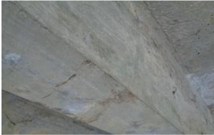
Figure 3-10: Shear cracks of deck slab at beam slab joint
