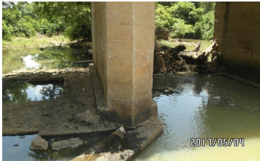
Figure 3-22: Weathering of cover concrete in a pier
