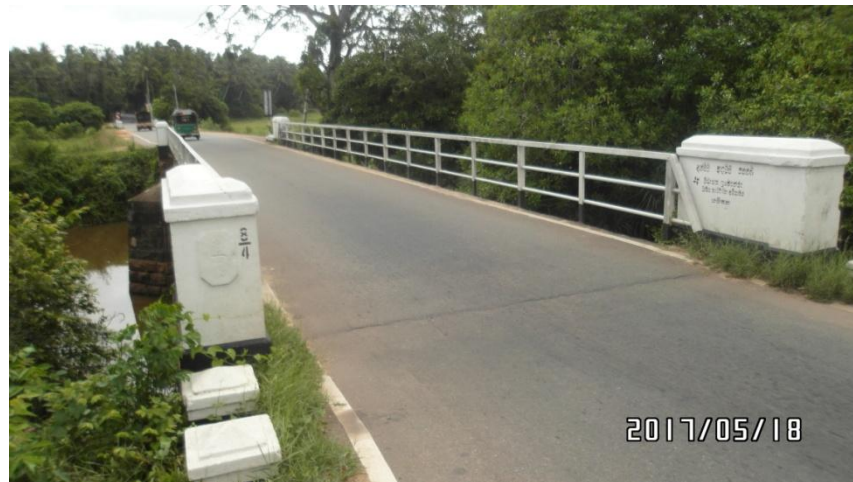
Figure 3-15: Cracking at an expansion joint, which is covered with asphalt
