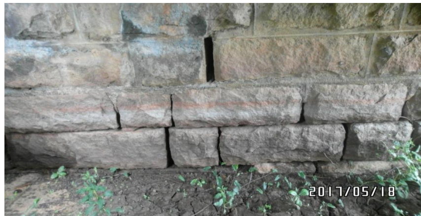
Figure 3-27: Mortar dislocation of a dressed stone abutment wall
