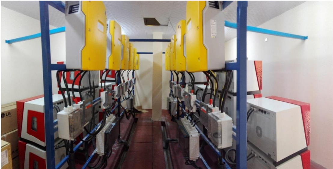
Figure 5.21: Battery backup system connected to the multi-cluster system.
