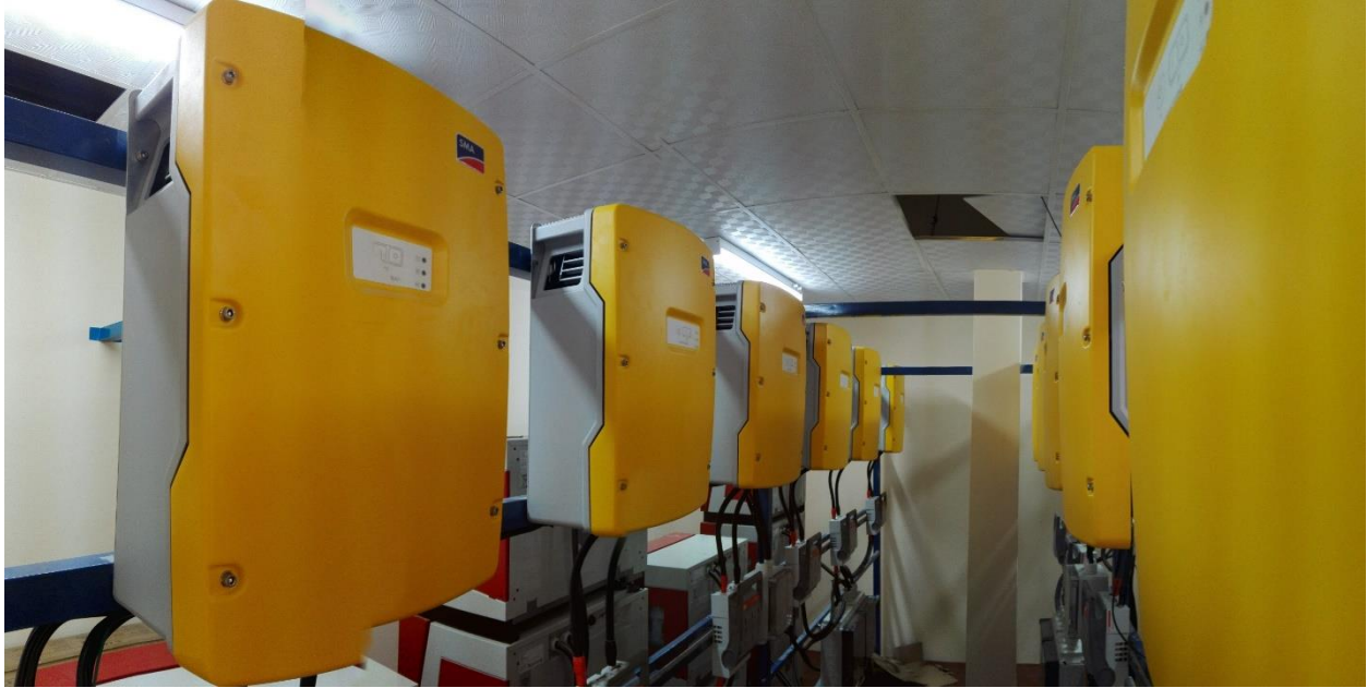
Figure 5.16: Sunny Island inverters operating at the site
