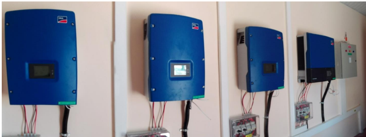
Figure 5.12: Solar inverters operating at the site
