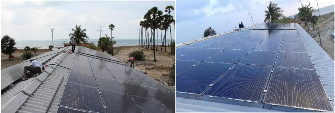
Figure 5.9: fixing solar modules on top of the powerhouse operating at the site.
