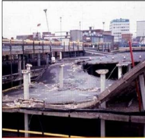
Figure 2.2- Brittle punching failure in flat slabs (source civildigital.com)
