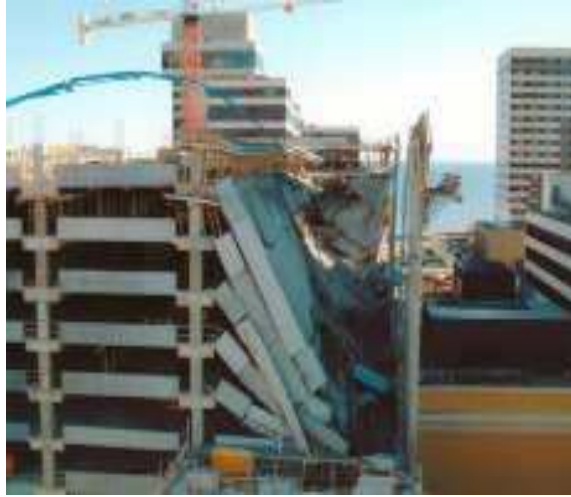
Figure 2.4-Flat slab failure an earthquake (Tropicana Casino Parking Garage)
