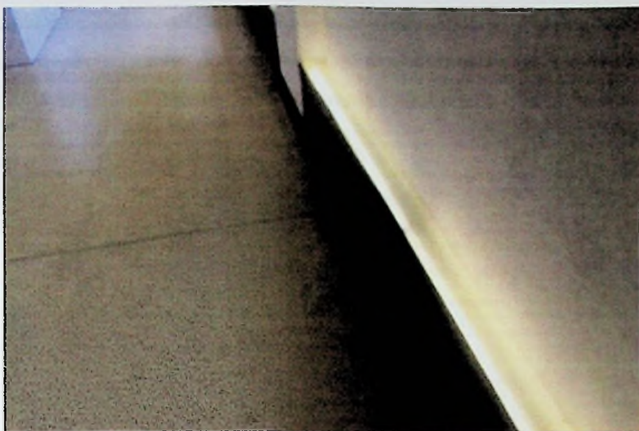
Figure 1.16: Crown spa and Salon – LED strip lights hidden inside skirting
