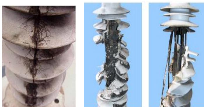
Figure 10: MOV arrester failure
