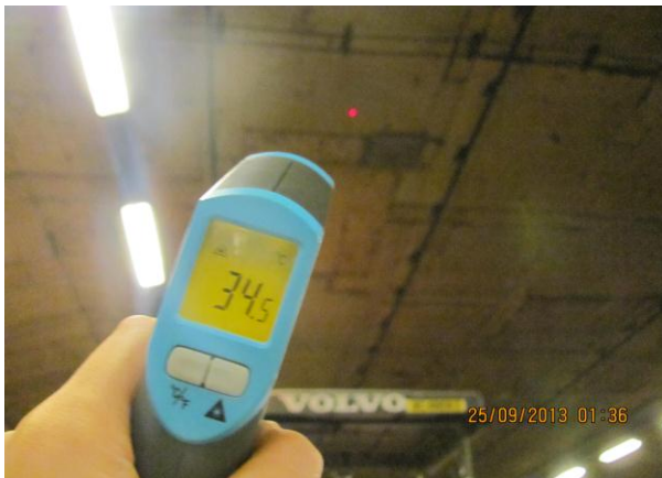
Temperature monitoring at the tunnel's ceiling
