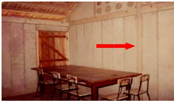
Figure 4-36: The removed column by the user thinking that 9 columns are inauspicious
