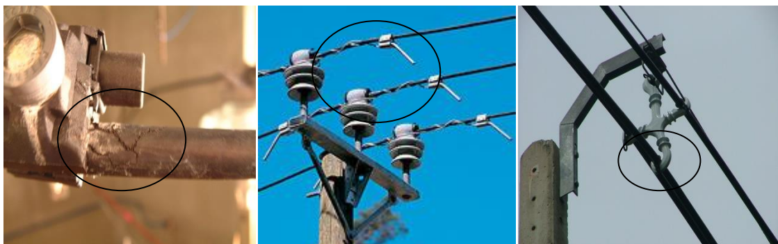
Figure 2-3: MV Covered Cable Damages at Supportive Points
