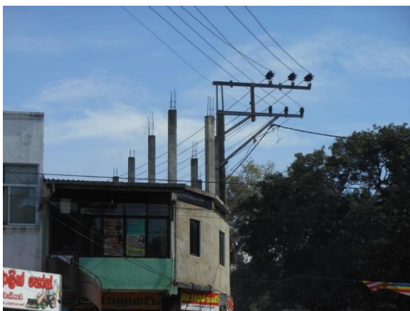
Figure 1-1: Inadequate Safety Clearance
