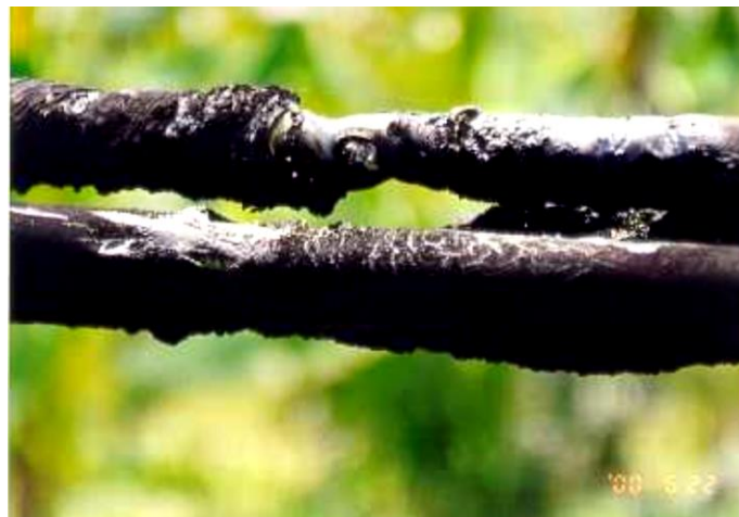
Figure 3-3: Burnt Outer Sheath
