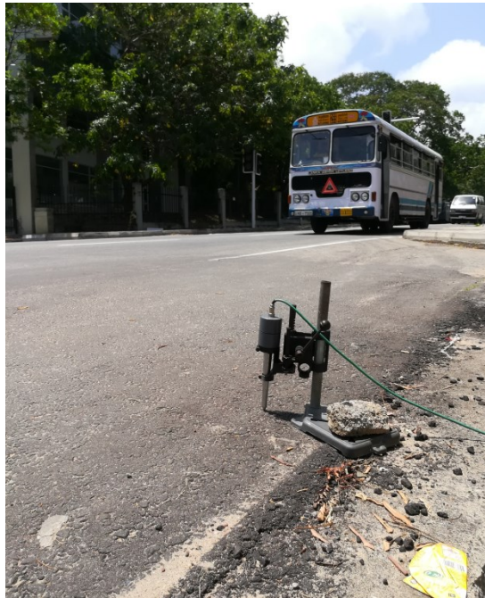
Figure 2.1 Sensor installed nearby the road
