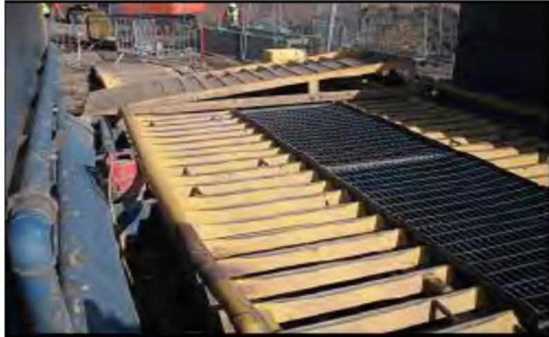
Figure 2.22: Drive On-Wheel Wash Area
