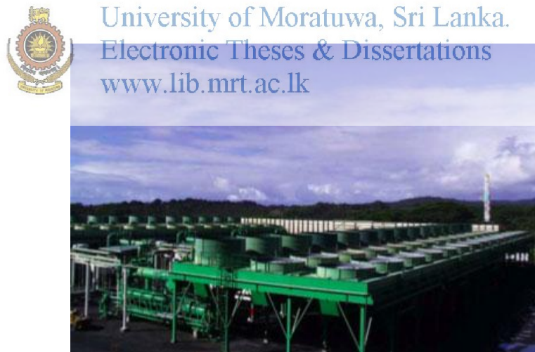
Figure 2.9: Combined cycle power plant installed in Hawaii, USA
