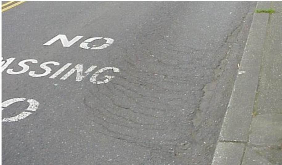
Figure 2-16: Slippage cracks (original in colour)
