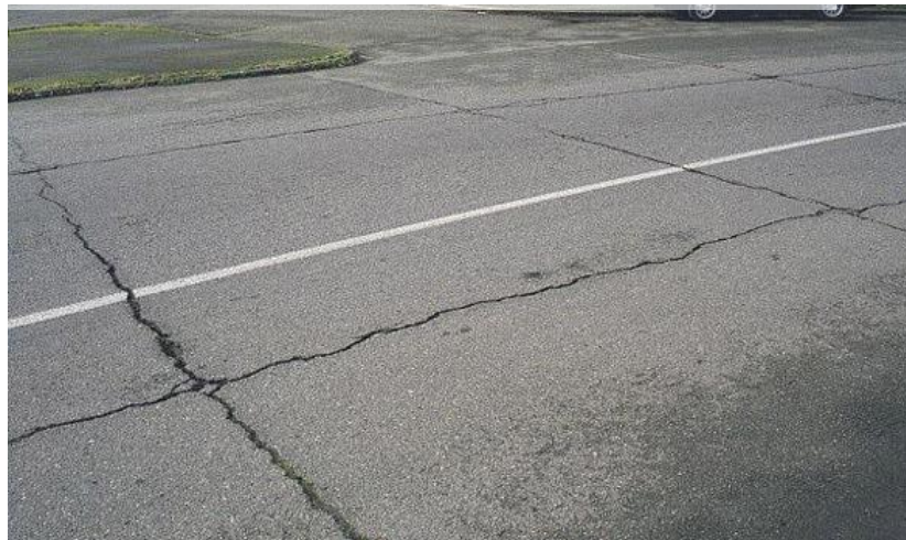
Figure 2-15: Joint reflection cracks (original in colour)
