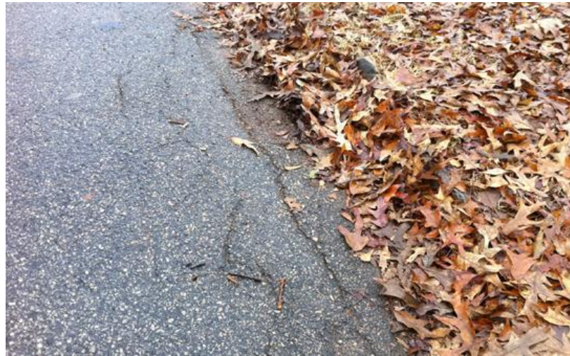
Figure 2-14: Edge cracks (original in colour)
