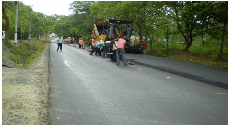
Figure 3-9: Laying of asphalt on a road which has HMA over lay 5 years before (original in colour)
