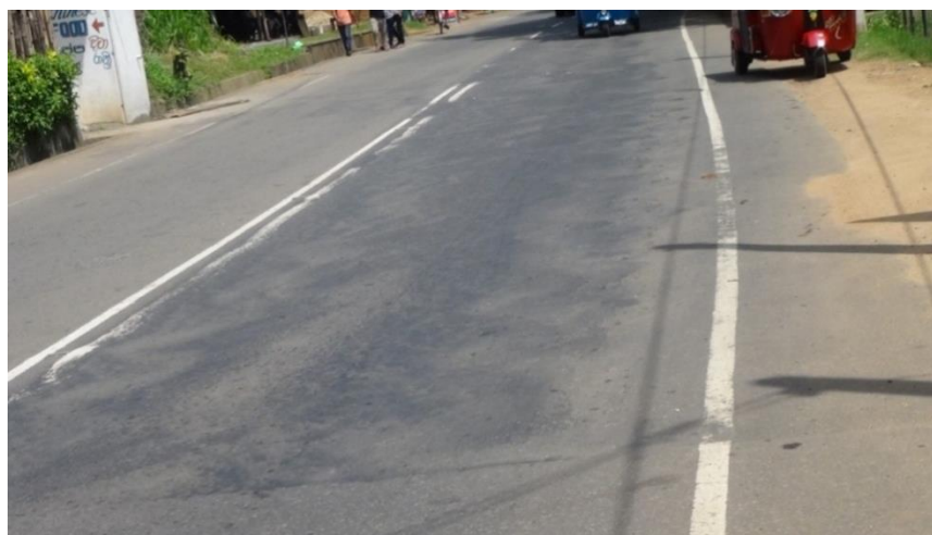
Figure 2-22: Bleeding (original in colour)
