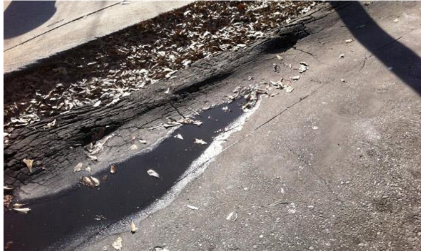
Figure 2-19: Rutting (original in colour)
