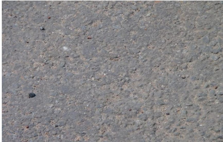
Figure 2-21: Raveling (original in colour)
