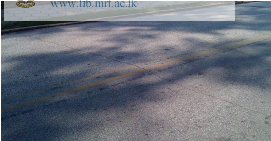
Figure 2-13: Transverse cracking (original in colour)
