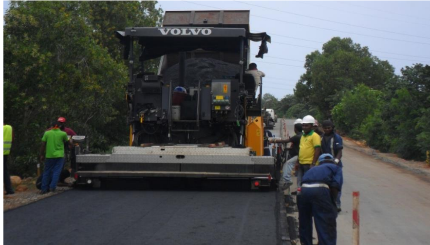
Figure 3-2: Asphalt laying on top of the complete base course (original in colour)
