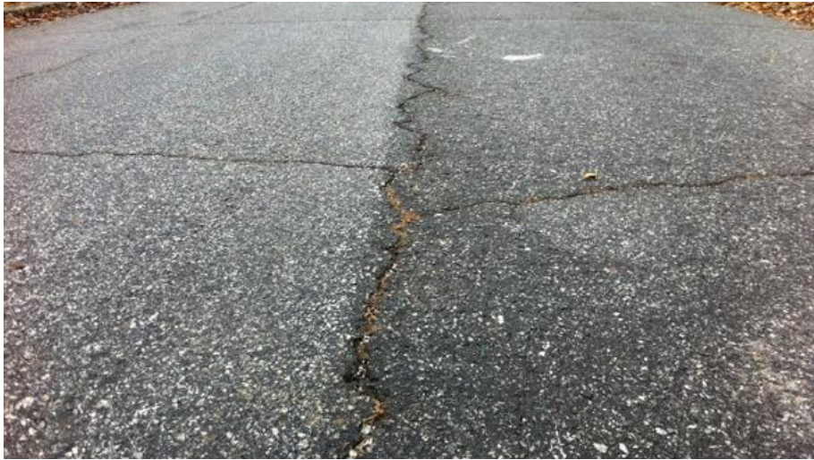
Figure 2-12: Longitudinal (linear) cracking (original in colour)
