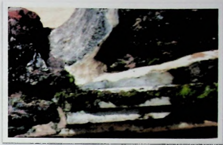
Moss and algae on lime plaster
