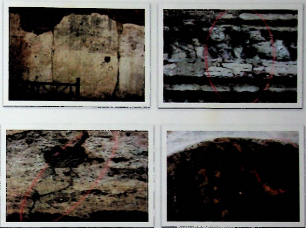
Cracks on the walls of Thivanka image house.
