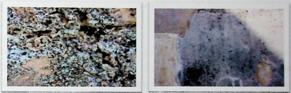
Moss and cracked growth on bricks and lime plaster
