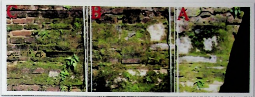
Botanical damages in foundation
