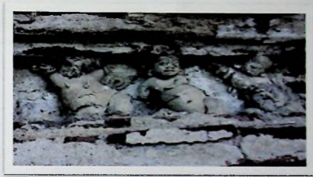
Gana (Dwarf) figures totally damages by thermal cracks.
