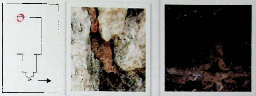
Damage caused by termites
