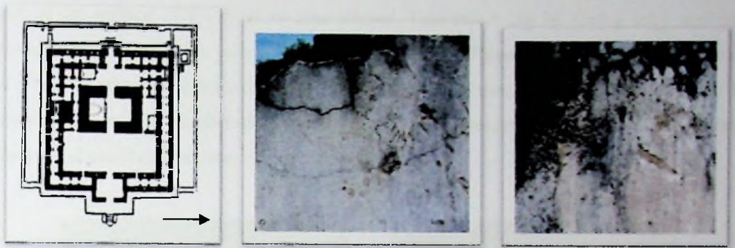
Small cracks on plaster
