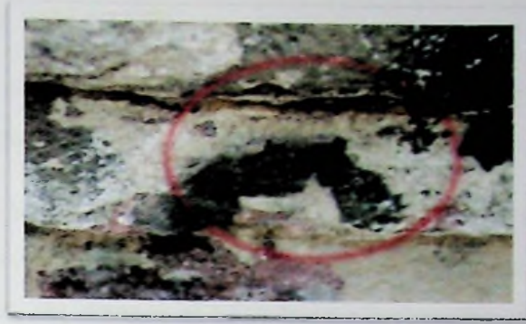
Peeling off of moss along with lime plaster.
