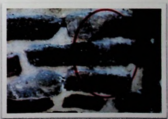
Small cracks on bricks
