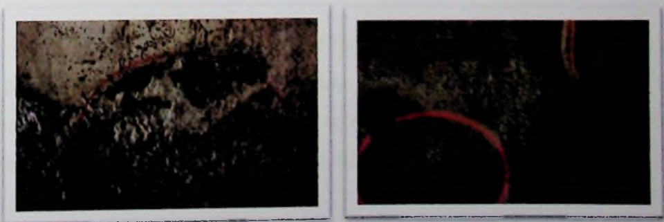
Deterioration of wall absorption of underground water
