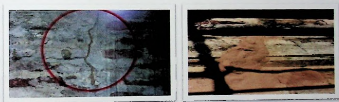
Termites on the base - Picture 110
