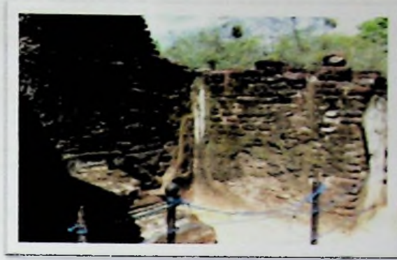
Deterioration of plaster Palace of king Parakramabahu
