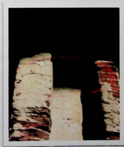
Micro cracks on the southern wall
