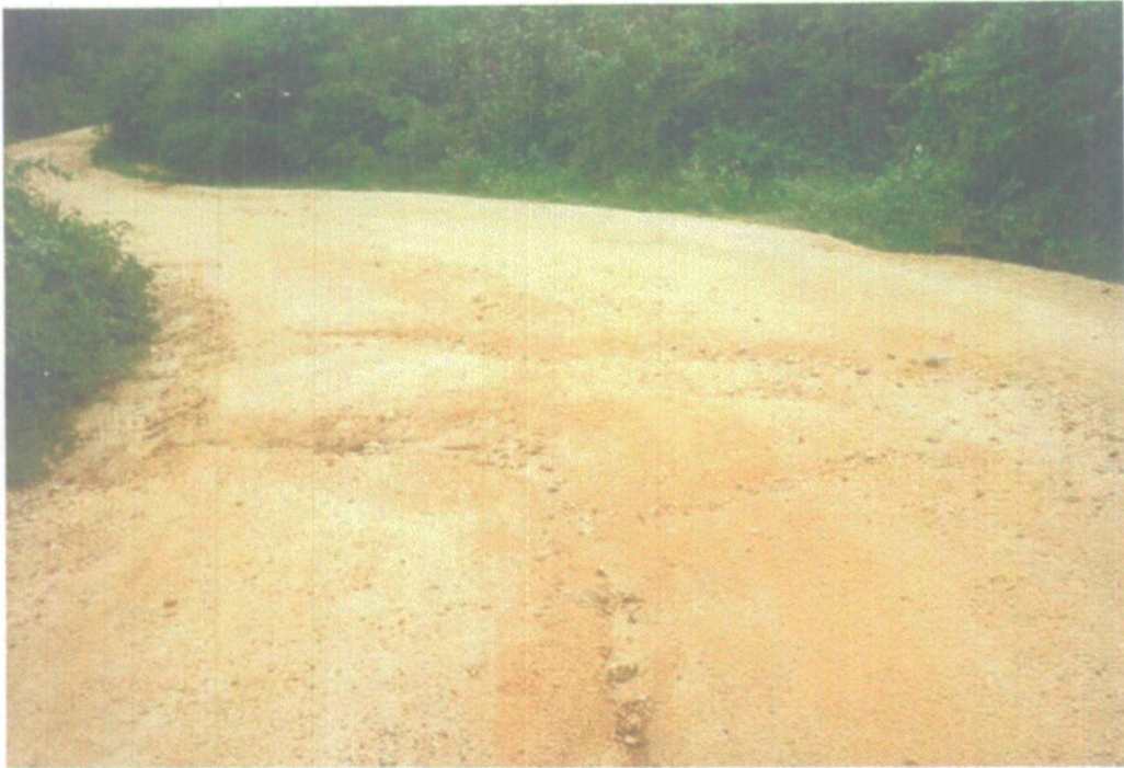
Figure 8.2 Erosion of carriageway and formation of gullies
