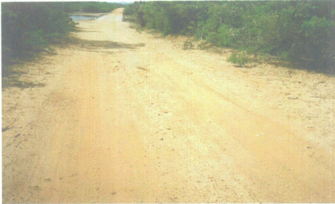
Figure 8.1 Wheel path rutting University of Moratuwa, Sri Lanka. Electronic Theses & Dissertations lib.mrt.ac.lk
