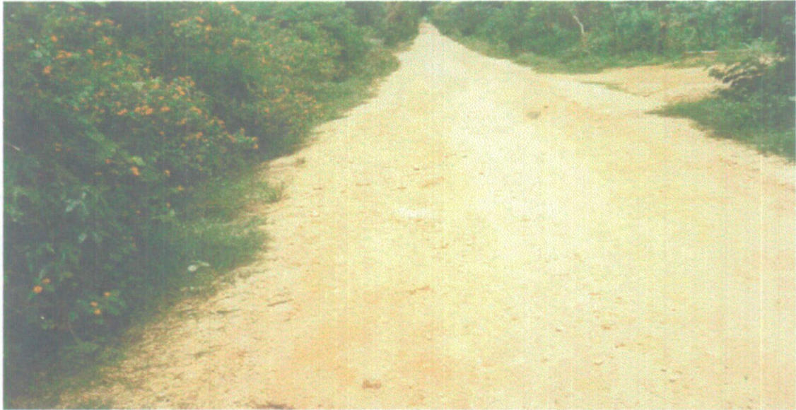
Figure 3.4 Erosion of embankment slope
